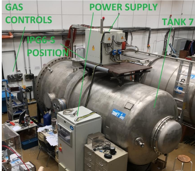
Fig. 4 IPG6-S refurbished facility
